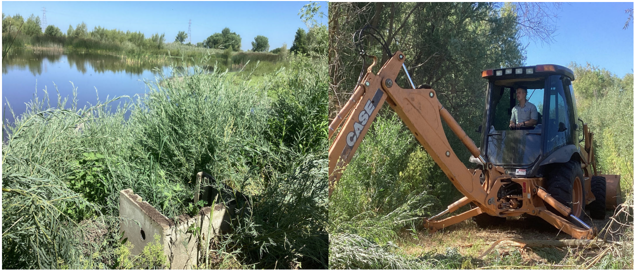
Image: Blocked culvert
